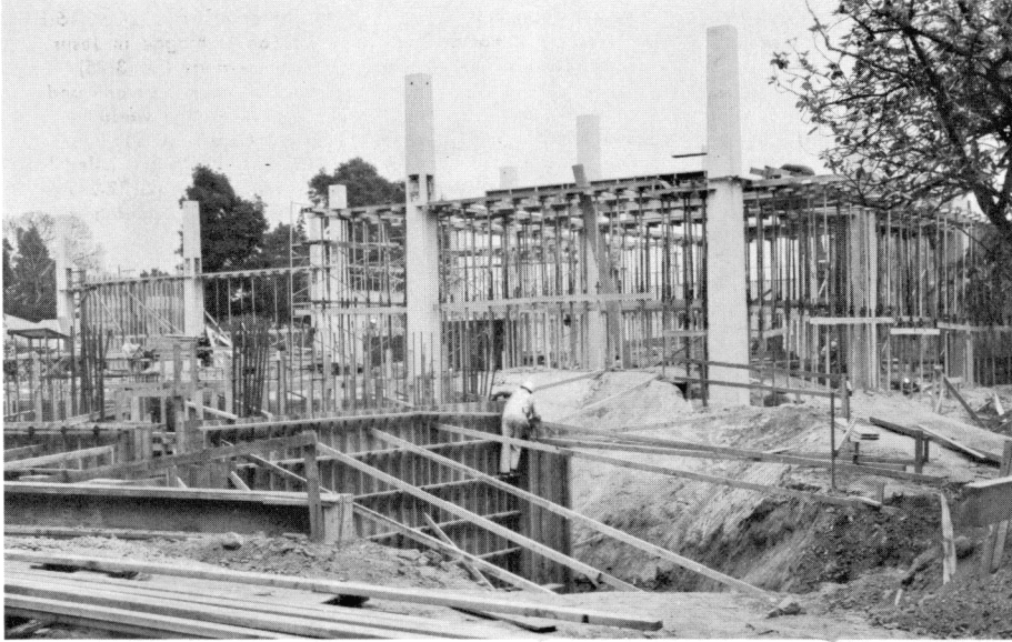
GOING UP —The pre-stressed concrete columns shown above will support an equal number of lightweight "umbrellas" of similar construction, which will become a part of the roof. The columns rest on foundational pillars extending 53 feet below ground level. Heavy-duty cranes will soon hoist the large roof beams—78 feet long—similar to those used in the gymnasium.
